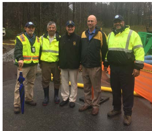
County Manager Dick Anderson visits pipe repair/rehab project in South Fulton in the early days of 2019.
